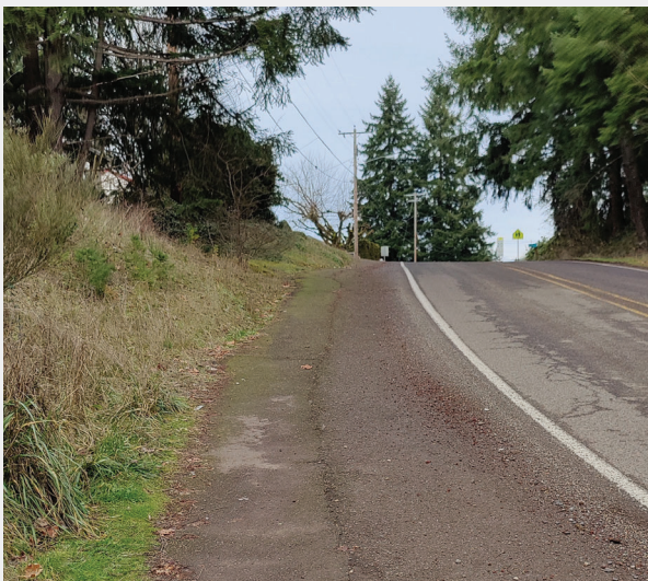
The shoulder on Mountain View Rd is paved in some locations, but in others, remains unpaved or is nonexistent.
