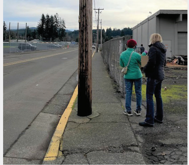
18th Ave has sidewalks on both sides south of Hwy 20 for much of its extent. However, in many places the sidewalk is narrow, sloped, and blocked by utilities or shows cracked or degrading panels.
