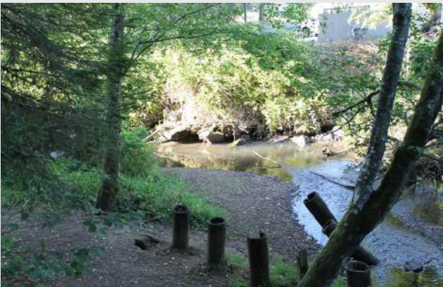
4. Significant bank erosion
