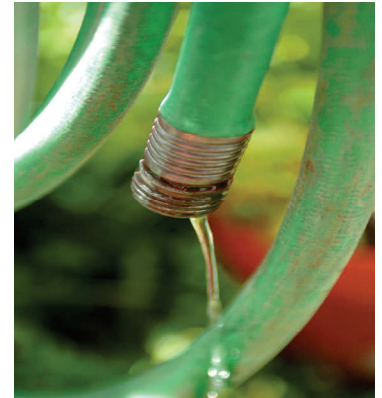
Leaking water hoses can be as wasteful as leaks inside the building.
