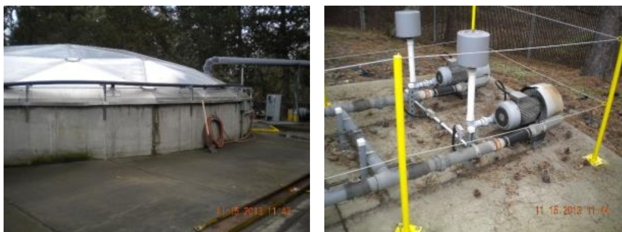
Figure 5-18. Solids holding tank exterior (left) and blowers (right)
