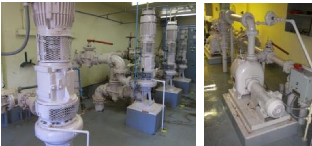
Figure 4-12. RAS pumps (left) and WAS pumps (right)
