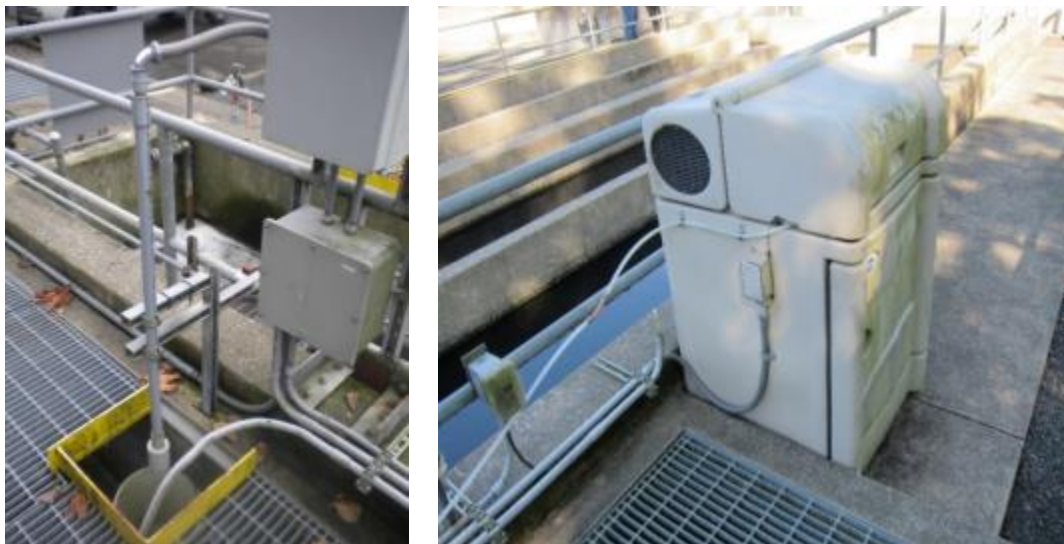
Figure 4-15. Effluent flow metering and sampling
