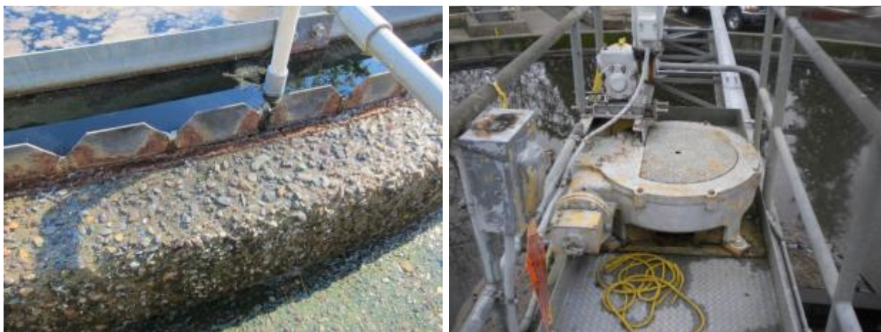
Figure 5-11. Original secondary clarifier weir (left) and drive mechanism (right)
