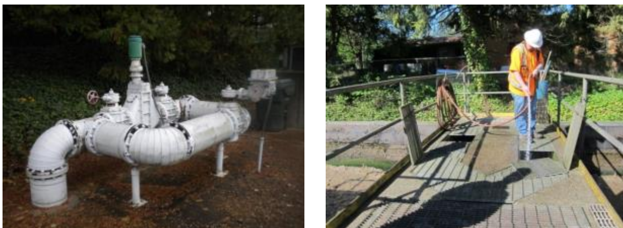
Figure 4-10. Influent grinder station (left) and manual bar screens (right)
