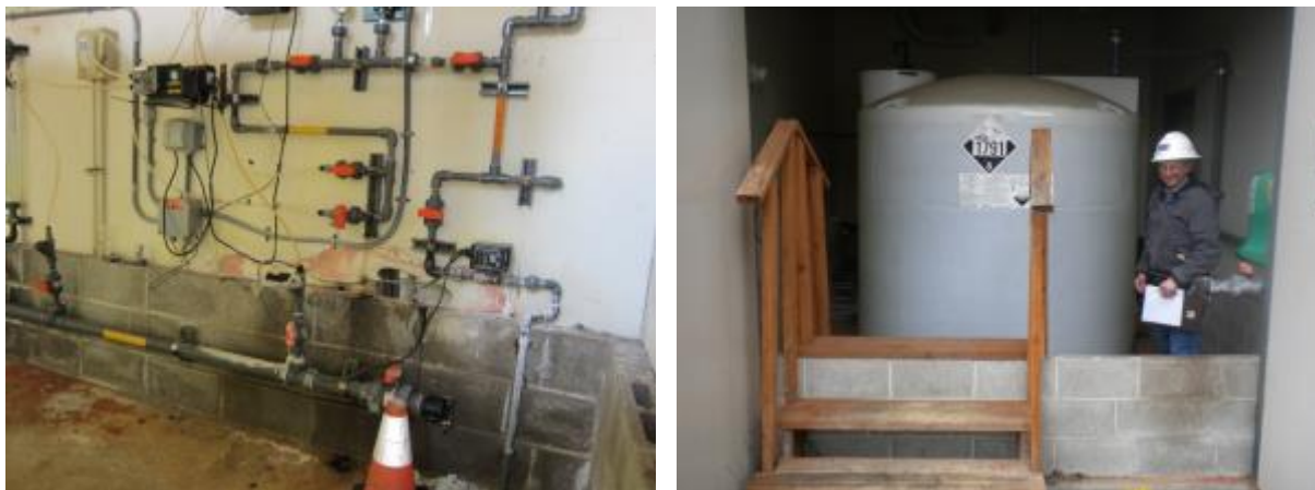
Figure 5-15. Sodium hypochlorite feed equipment (left) and storage tank in containment area (right)
