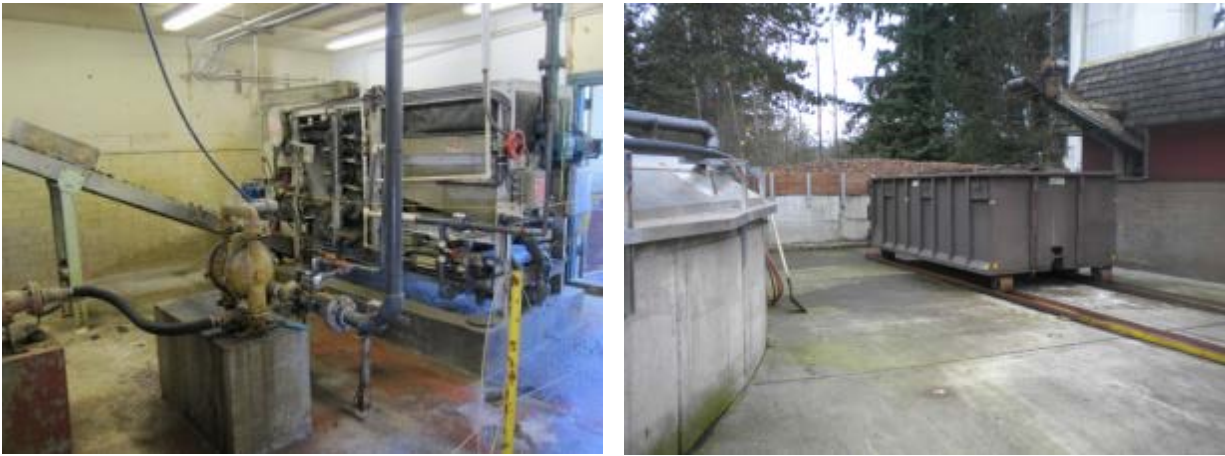
Figure 4-20. Dewatering room interior (left) and exterior (right) with 20 yd 3 container on rails
