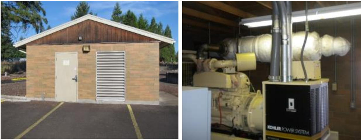
Figure 4-17. Standby generator building (left) and equipment (right)
