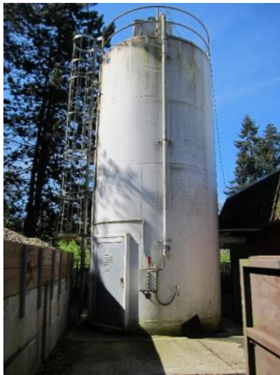
Figure 4-22. Lime silo adjacent to solids handling building
