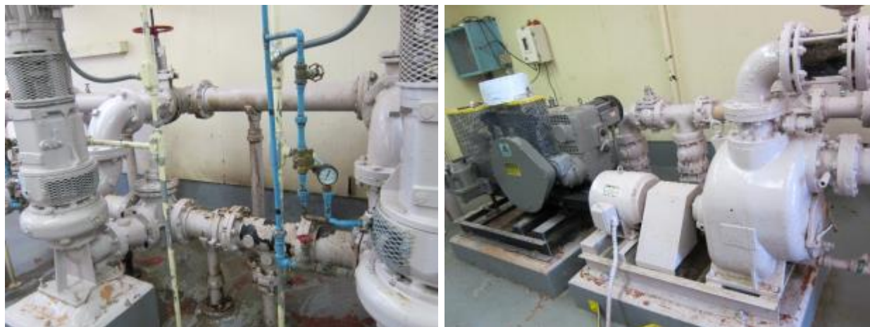
Figure 5-12. RAS (left) and WAS (right) pumping equipment
