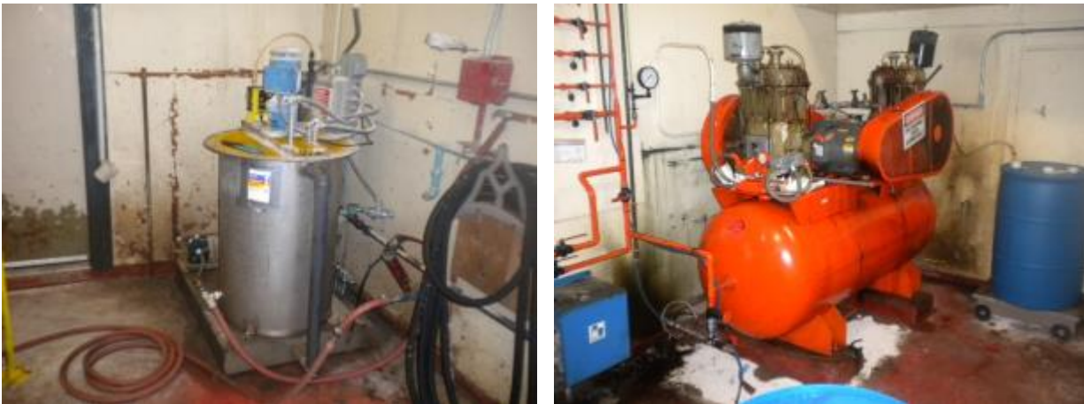
Figure 4-21. Polymer feed equipment (left) and plant compressor (right)
