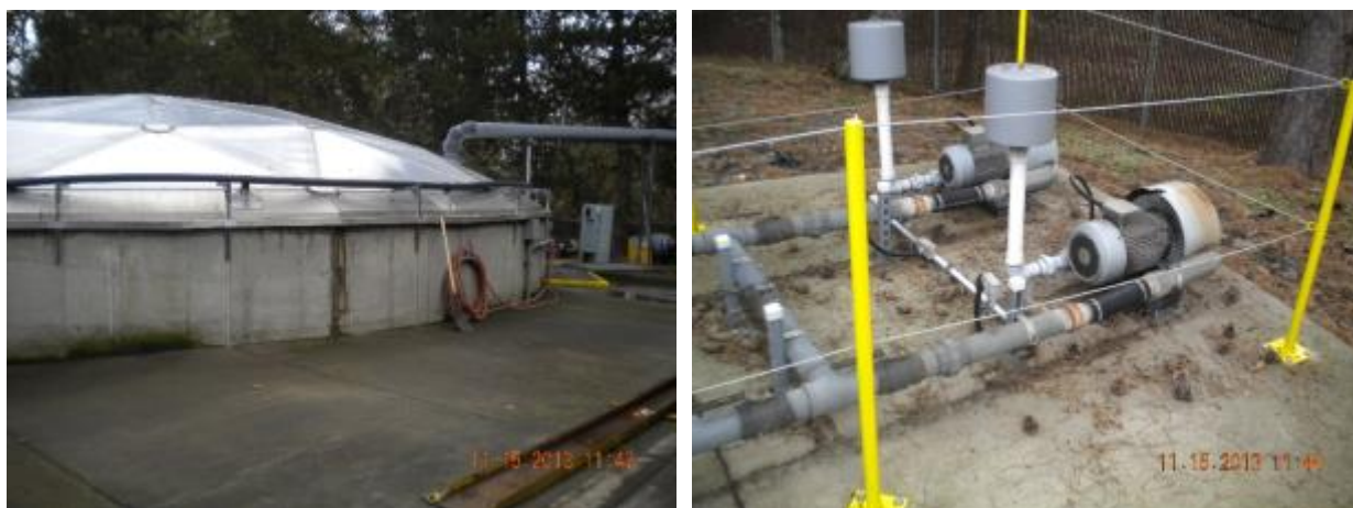
Figure 4-19. Covered solids holding tank (left) and mixing blowers (right)
