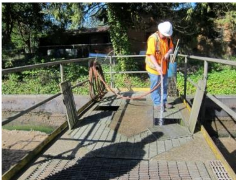
Figure 5-8. Routine cleaning of headworks bar screens
