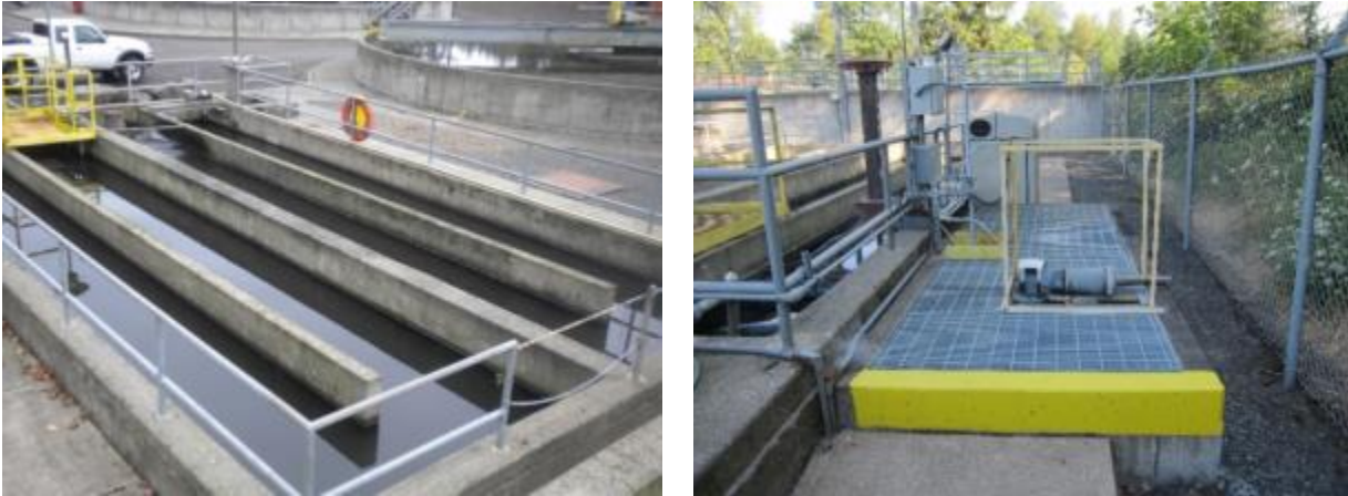
Figure 4-14. CCT (left) and effluent structure with chemical mixer (right)
