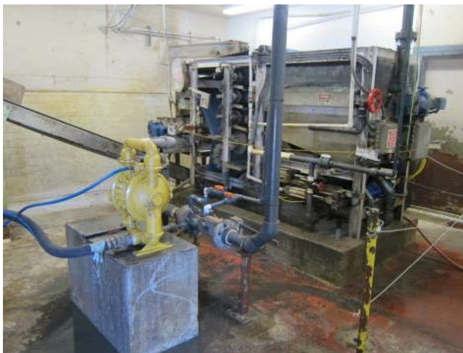
Figure 5-19. Solids feed pump, BFP, and conveyor
