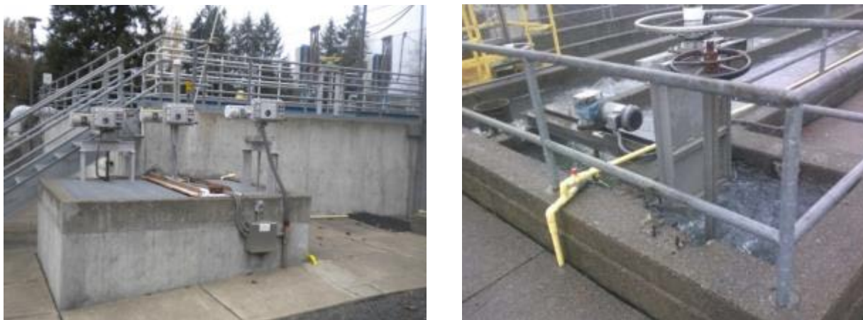
Figure 5-13. Secondary flow distribution structure (left) and CCT flow distribution box (right)
