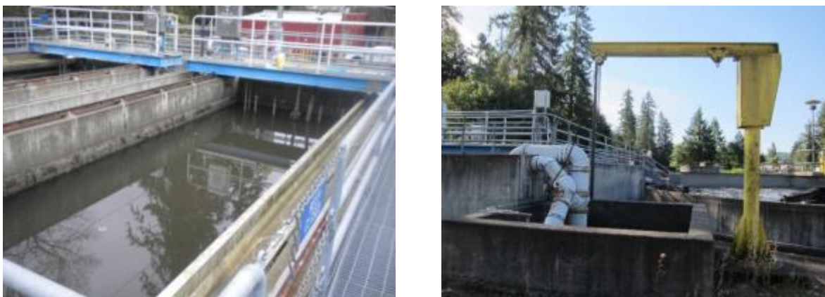
Figure 4-13. Traveling-bridge sand filters (left) and filter pump station (right)
