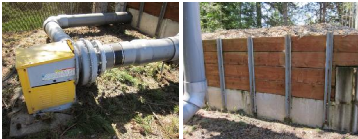
Figure 4-23. Odor control blower (left) and odor control biofilter (right)
