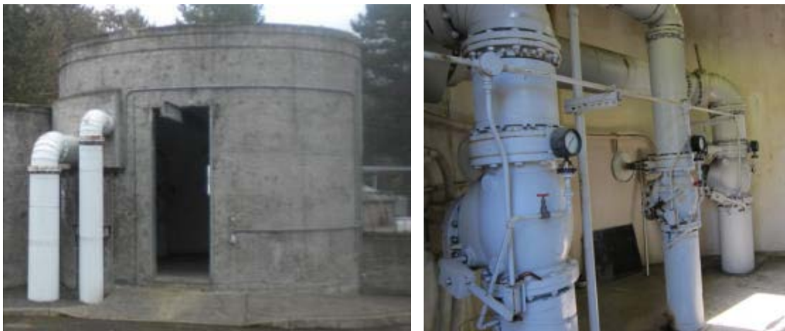
Figure 4-8. IPS exterior and dual force mains (left), and interior above-grade discharge piping (right)
