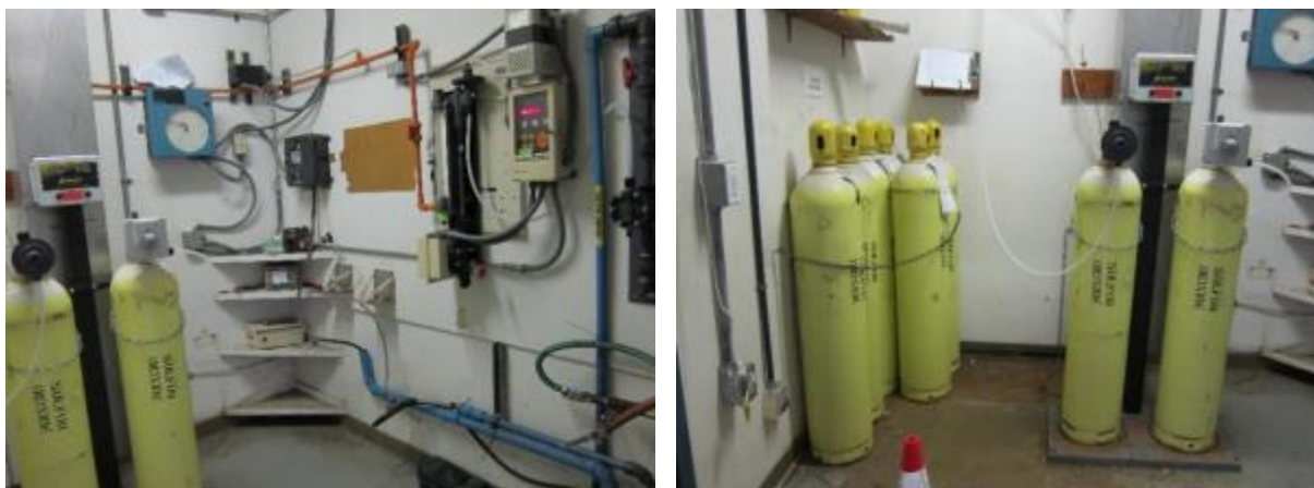
Figure 5-16. Sulfur dioxide feeding and analytical equipment
