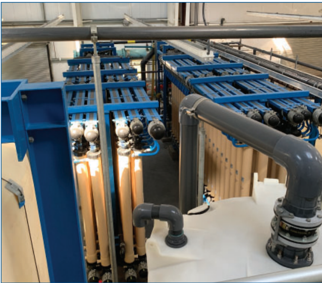
West Yost's team recently assisted the City of Cottage Grove in the design and construction of an expansion of the City's Row River membrane water treatment facility.
