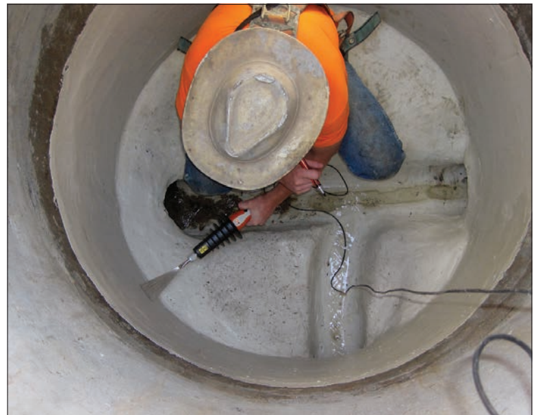
Dale Jarvis from subcontractor K&R Plumbing performs an electro test on an Epoxytec manhole liner.
