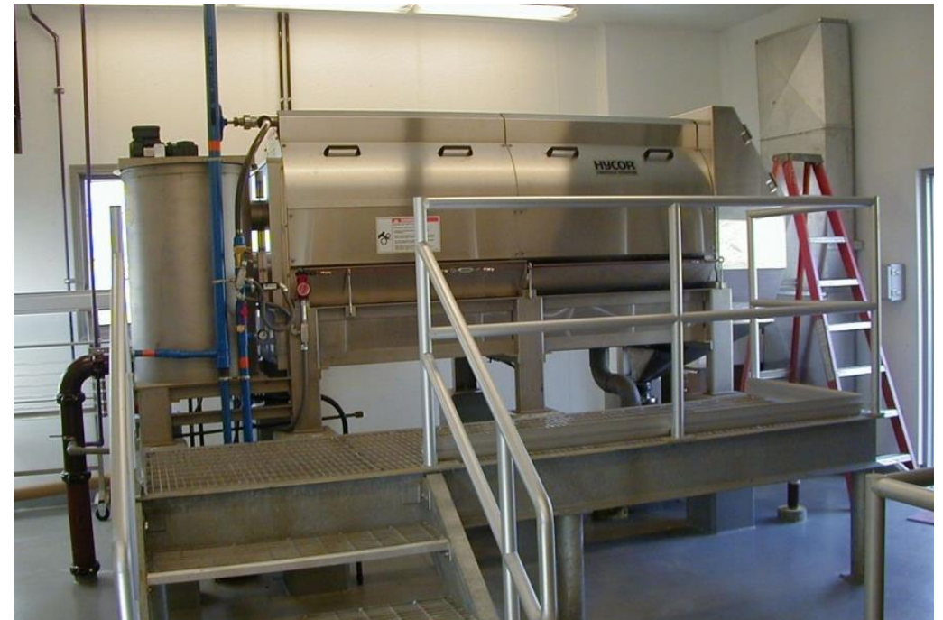
Install Sludge Thickening Equipment
